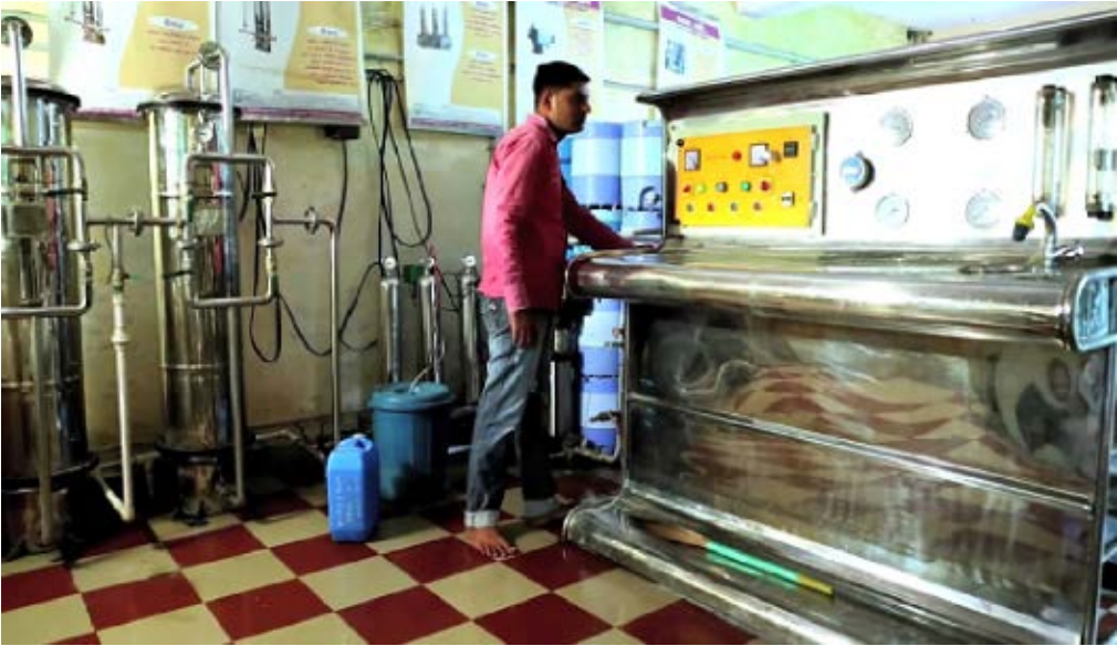
Picture 2.3: RO plant at Pansari, Gujarat
