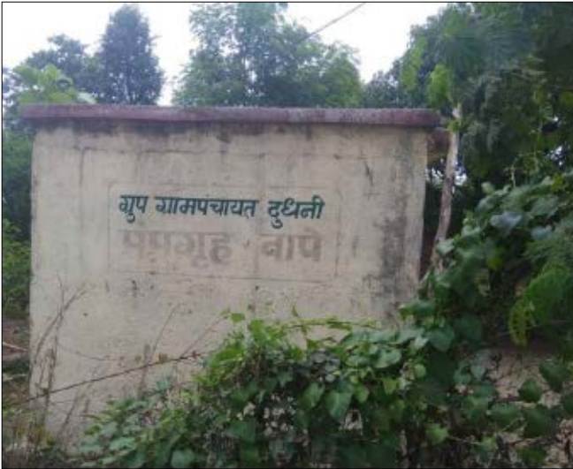
Figure 3C.7: Outside and inside view of pump house
