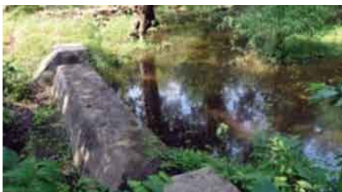
FIGURE 10 GULLY PLUG IN GHATA VILLAGE
