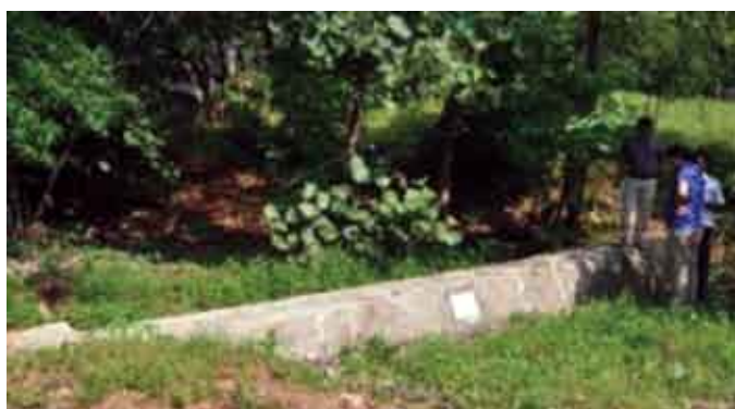
FIGURE 9 CHECK WALL IN GHATA VILLAGE
